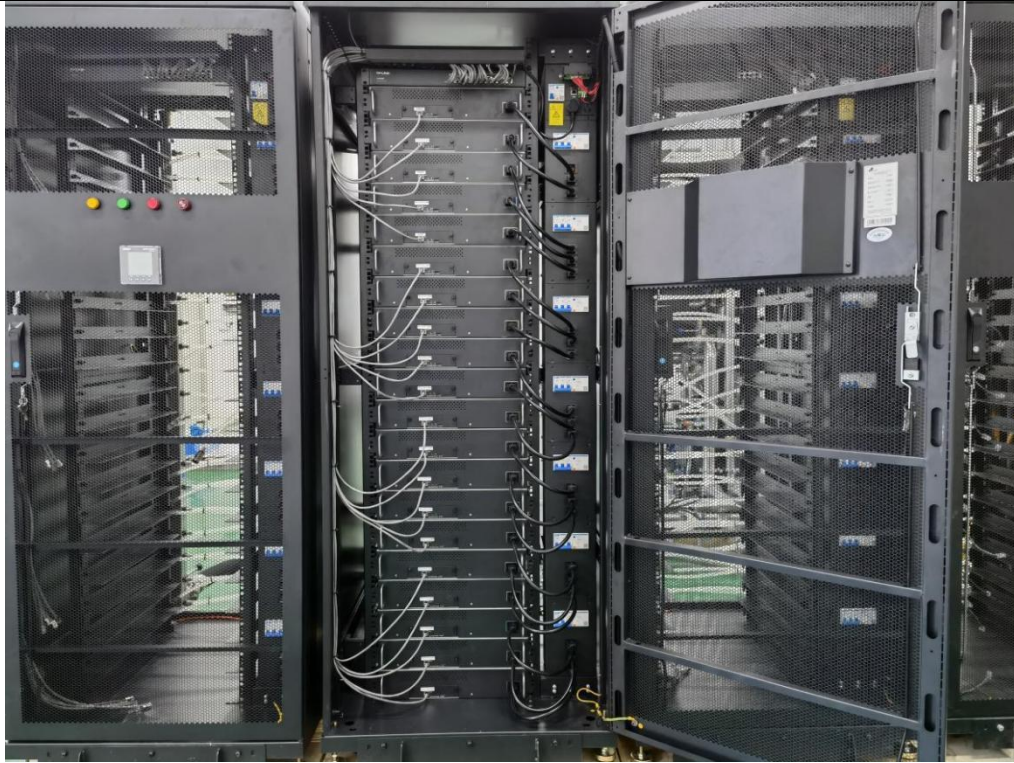
Front of the rack
